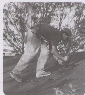
▲ fix the roof
